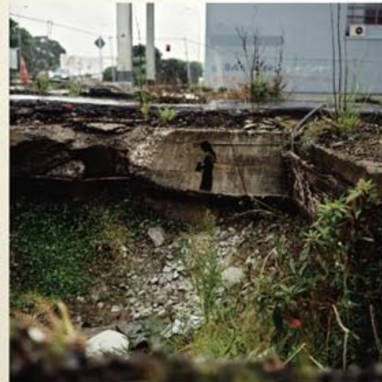
Petrol Pit An old overgrown hole in the ground which used to contain a petrol tank. Even this truck concrete can't keep nature at bay. Kingsland, Auckland
